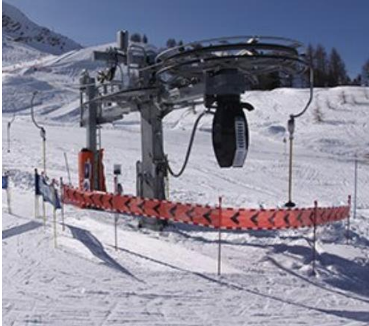
Figure 11: Surface Lift station
