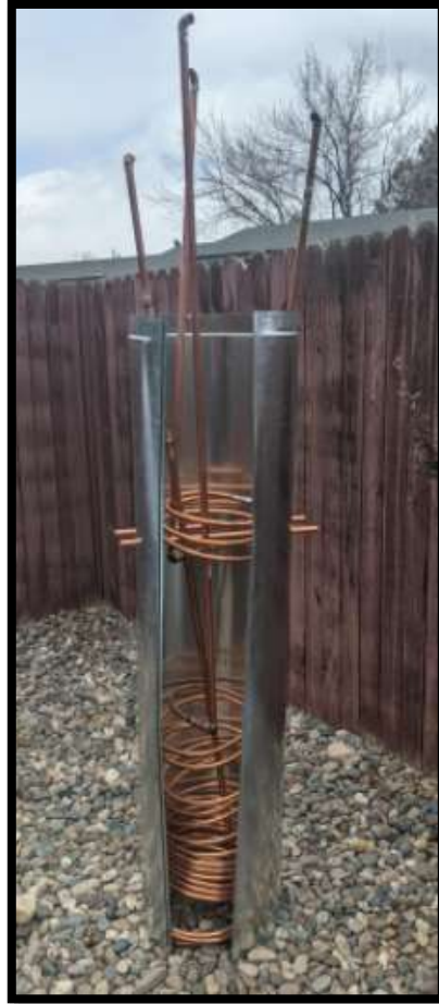
Figure 8: Heat exchanger ducting
