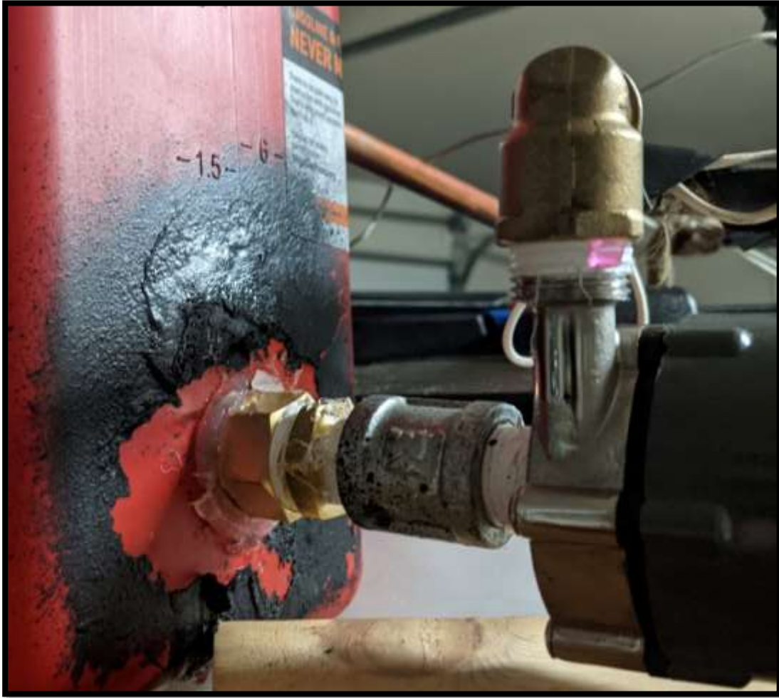
Figure 12: Pump connection to reservoir
