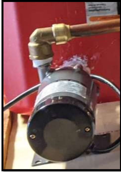
Figure 13: Pump fitting to heat exchanger
