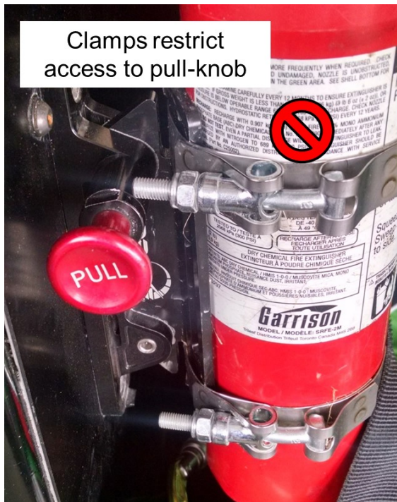
Figure B-46: Incorrect orientation of extinguisher clamps.
