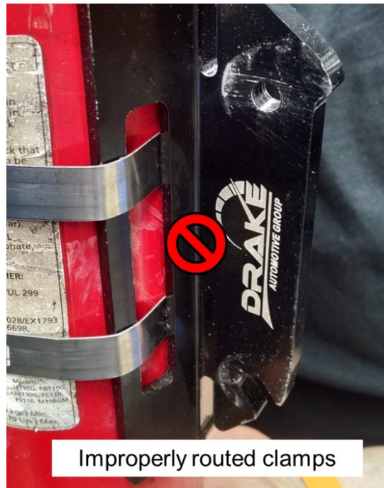
Figure B-47: Incorrect routing of hose clamps.
