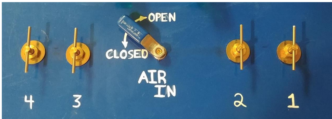
Figure 19: Pressure Measurement Control Valves
