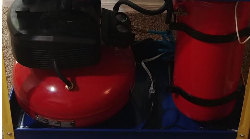
Figure 6: Air Compressor and Tanks
