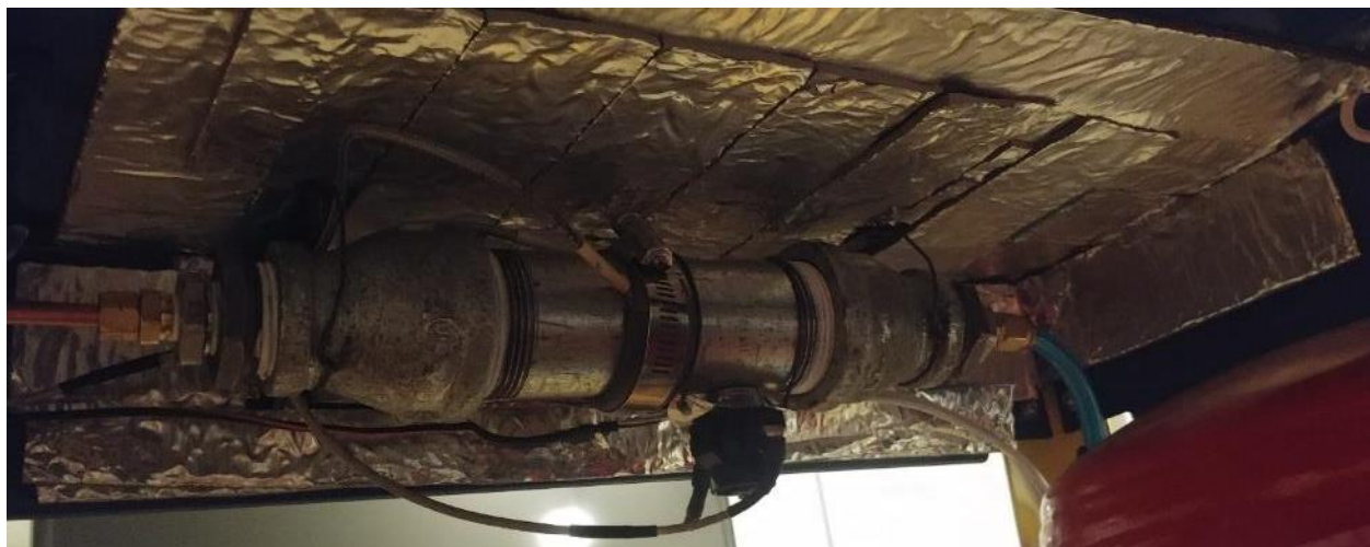
Figure 41: Heat Exchanger Mounted
