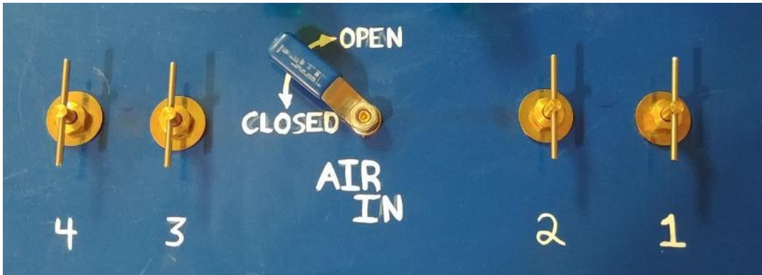
Figure 55: Pressure Measurement Control Valves
