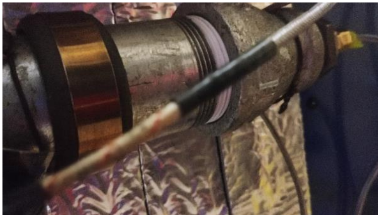
Figure 64: Heat Exchanger Wiring
