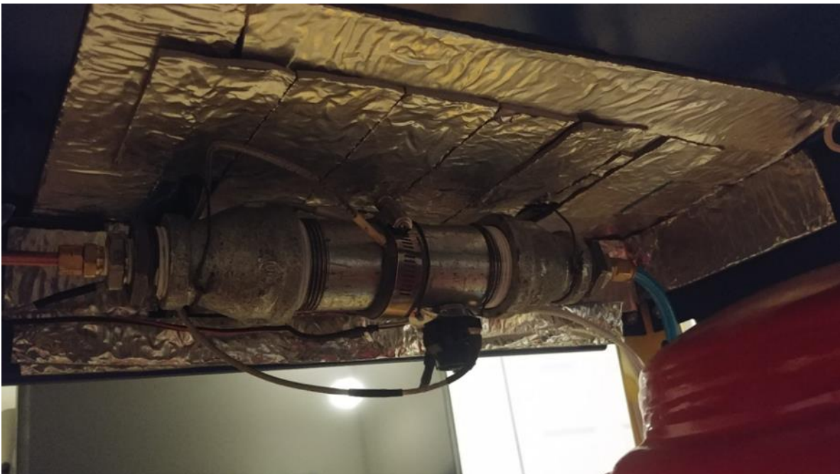
Figure 62: Heat Exchanger Insulation
