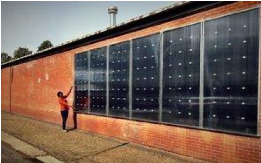
Figure 10: SolarThermiX Solar Air Heater on RTC Building
