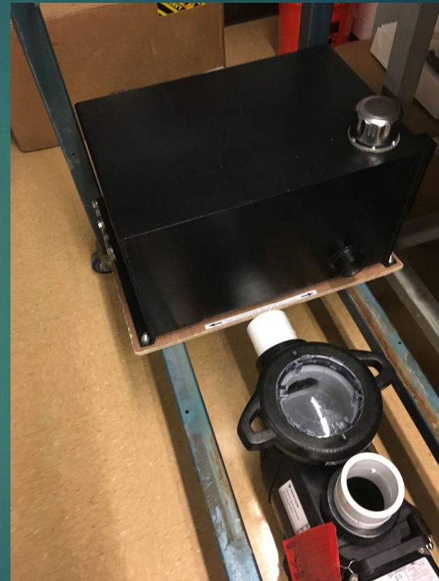
Figure 3 – Tank and Pump
