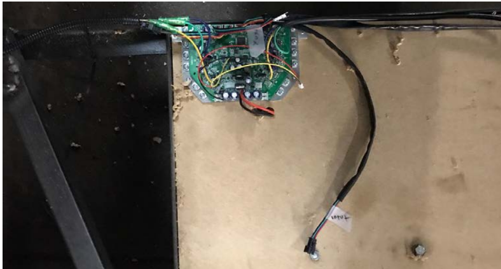
Figure 7: Electric board + wiring
