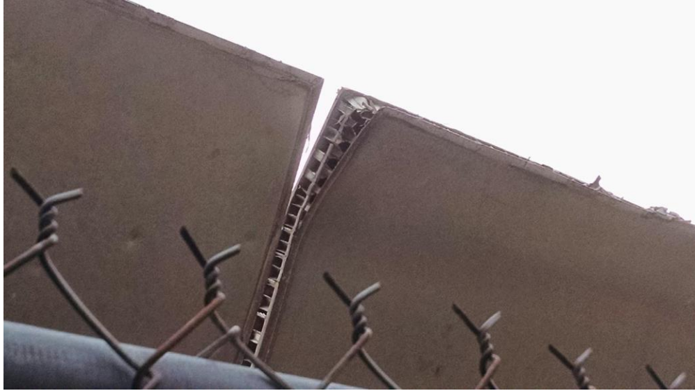
Figure 7 - Bent corner of trough
