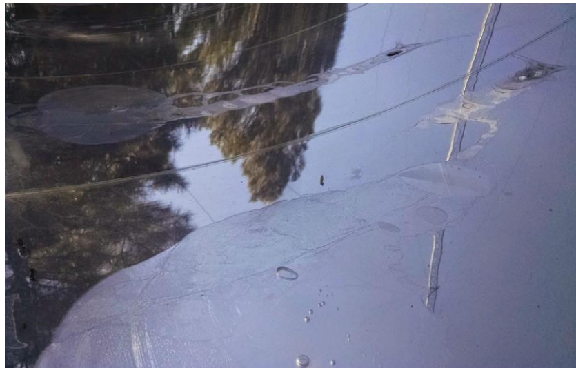
Figure 10 - Holes and water damage in surface
