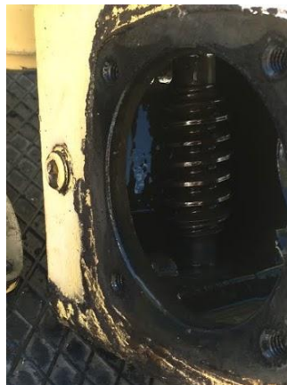
Figure 6: Vertical worm gear connecting the upper level to the lower level gearbox.
