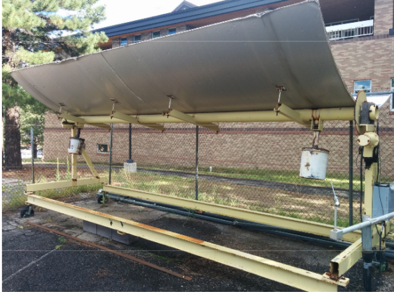
Overall picture of the system
