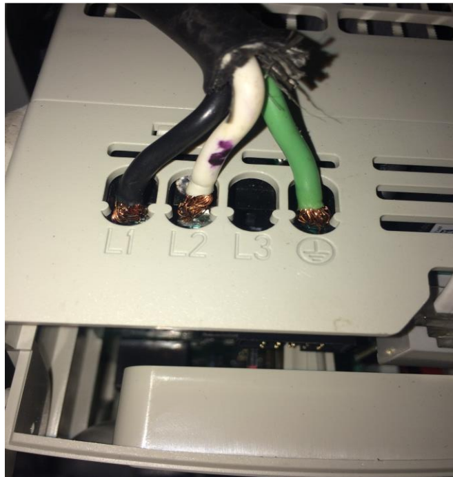
Figure 3- Drive power supply
