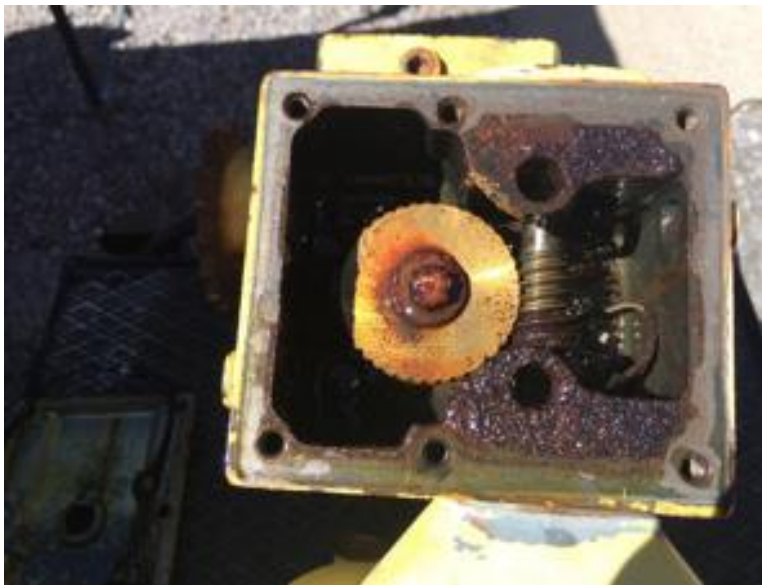
Figure 11- Upper gearbox with the cover off
