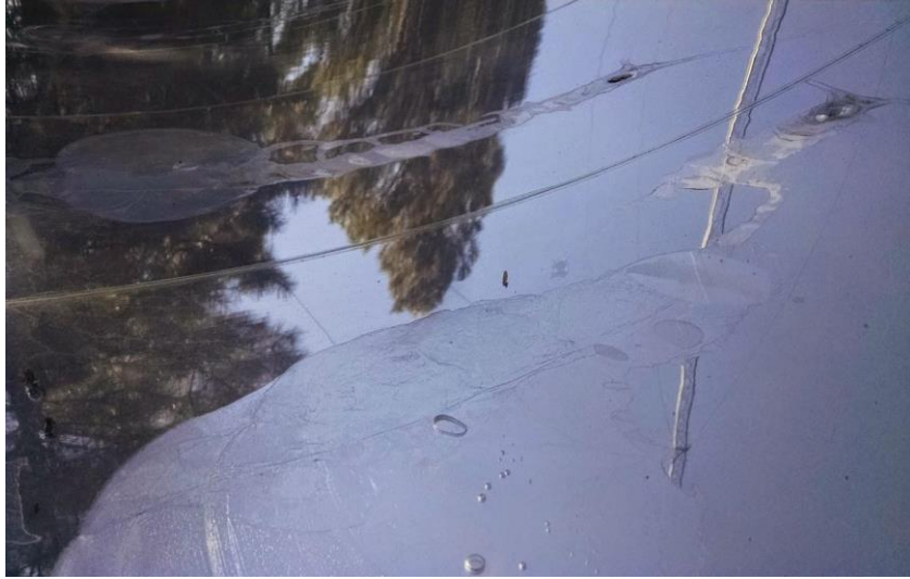
Figure 19 - Holes and water damage in surface
