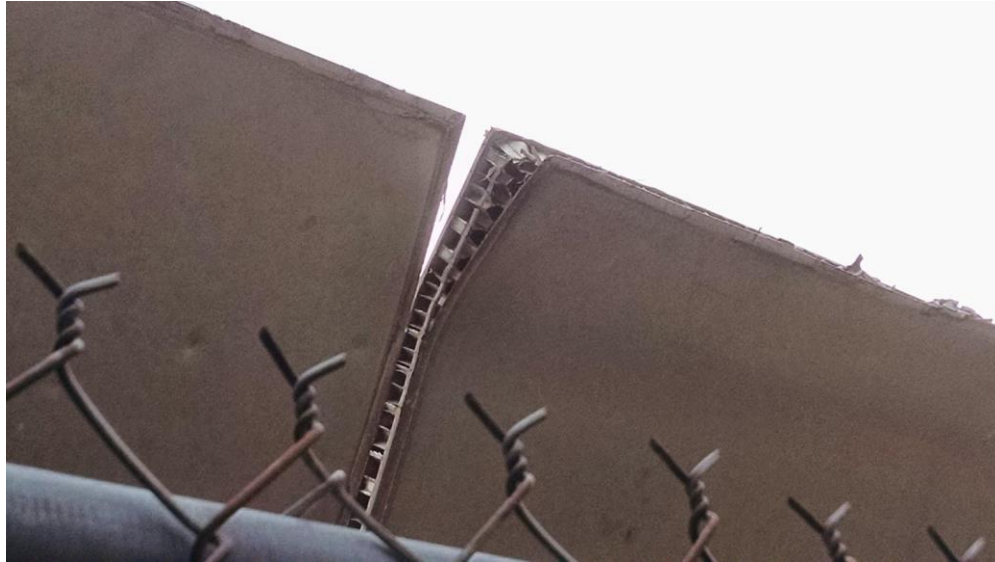
Figure 17 - Bent corner of trough
