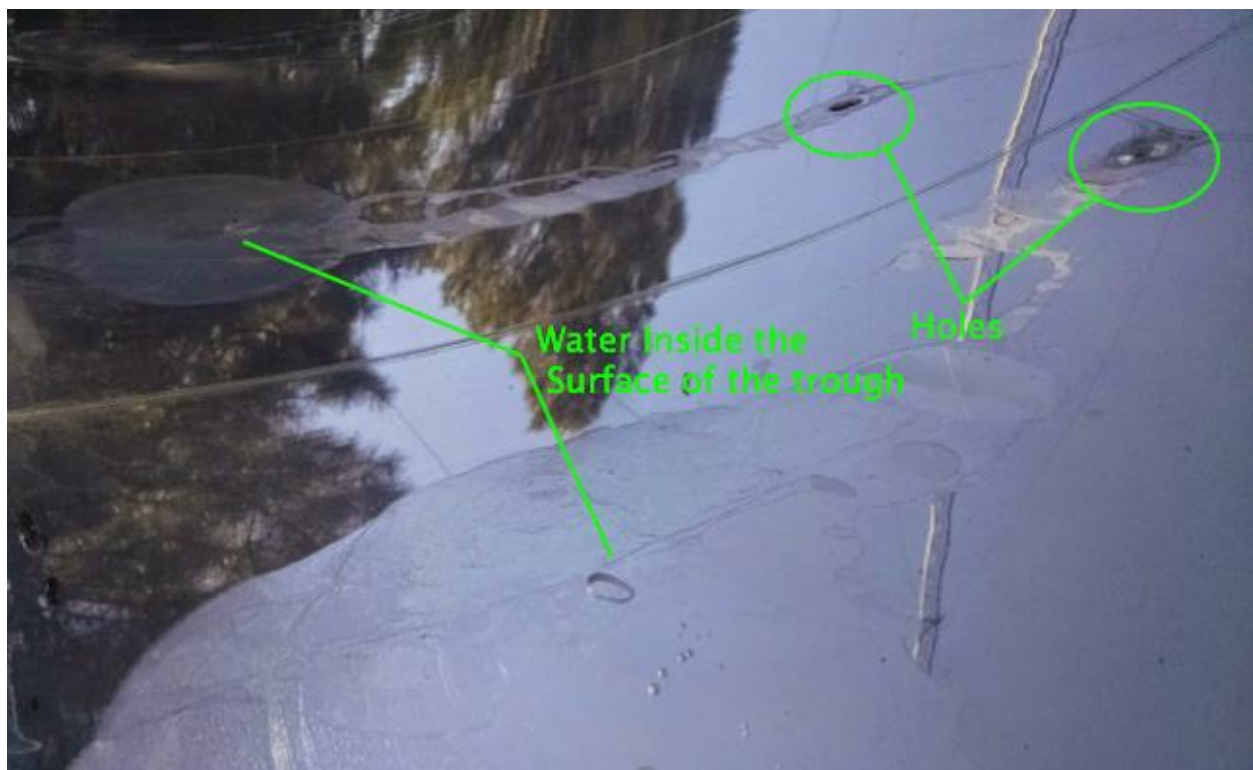
Figure 16 - Holes and water damage in surface
