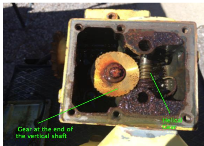
Figure 6 - Upper gearbox with the cover off
