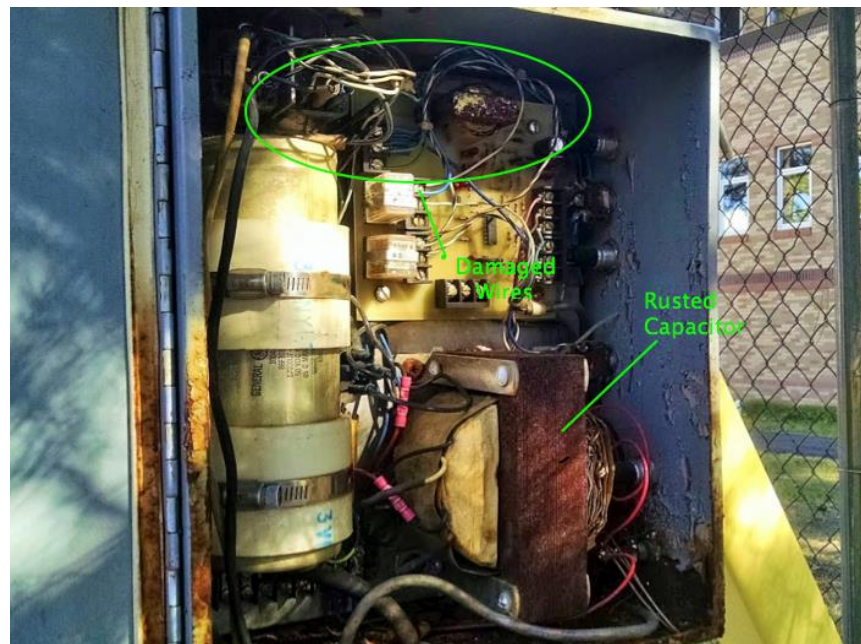
Figure 21 -Previous control box
