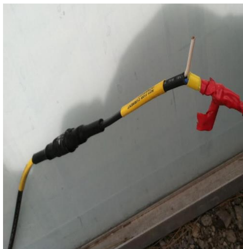
Figure 5.11: Solar panel negative end connection
