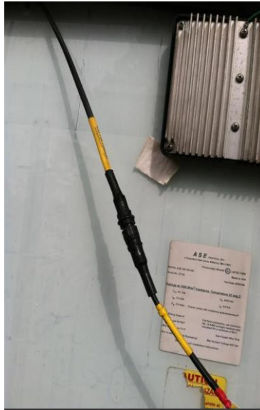
Figure 5.10: Solar panel positive end connection
