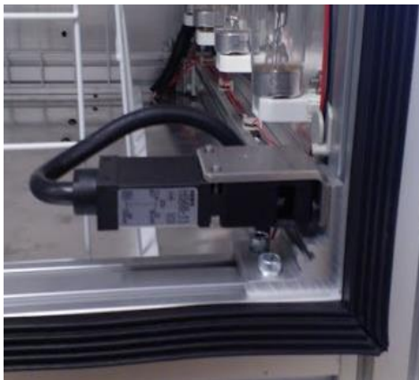
Figure 4.4: Door safety switch
