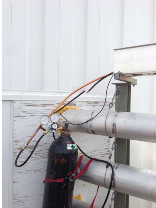
Figure 2.2.1- Nitrogen tank installed near astrometric hut.
