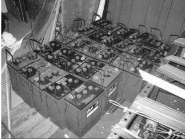
Figure 2.4. :Surrette S460 battery bank, 6 volts, 460 amp hrs
