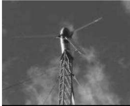
Figure 2.3.2. : 1.5 kW Bergey wind turbine
