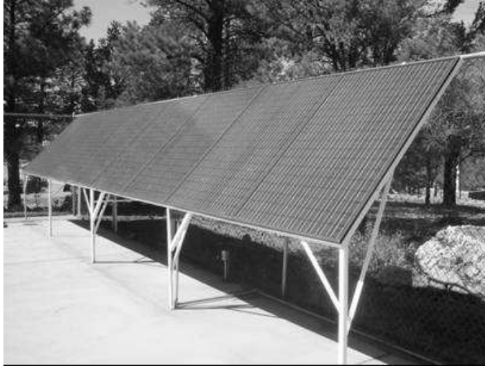
Figure 2.3.1.b. : PV cells of the 45° south-facing array
