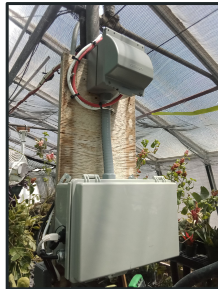
MAQ20 system installed in greenhouse
