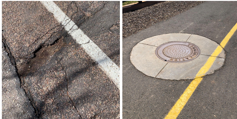
Figure 16: Left image is a crack, and the right image is a utility hole
