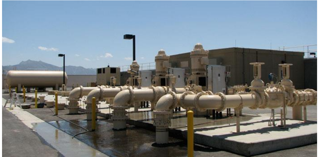
Figure 10: Rainbow Valley Water Treatment Facility [9]
