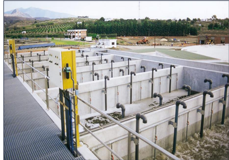
Figure 16: Sand Filter Example [16]
