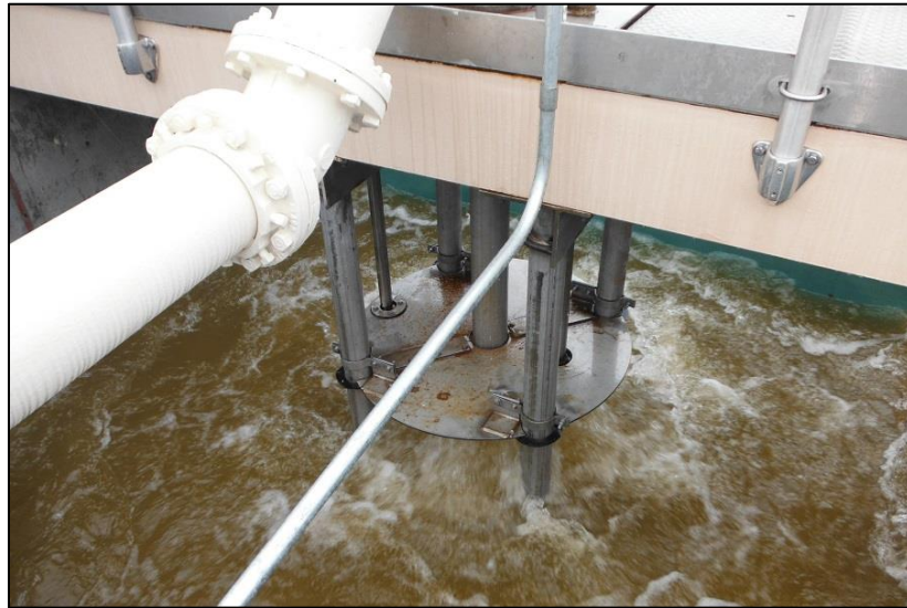
Figure 5. 6 Aerated Grit Chamber [28]
