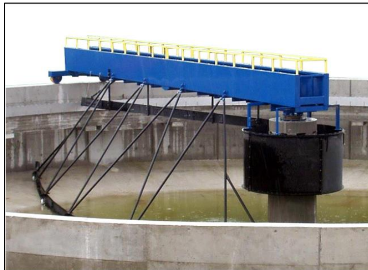
Figure 5. 11 Traction Primary Clarifier [33]
