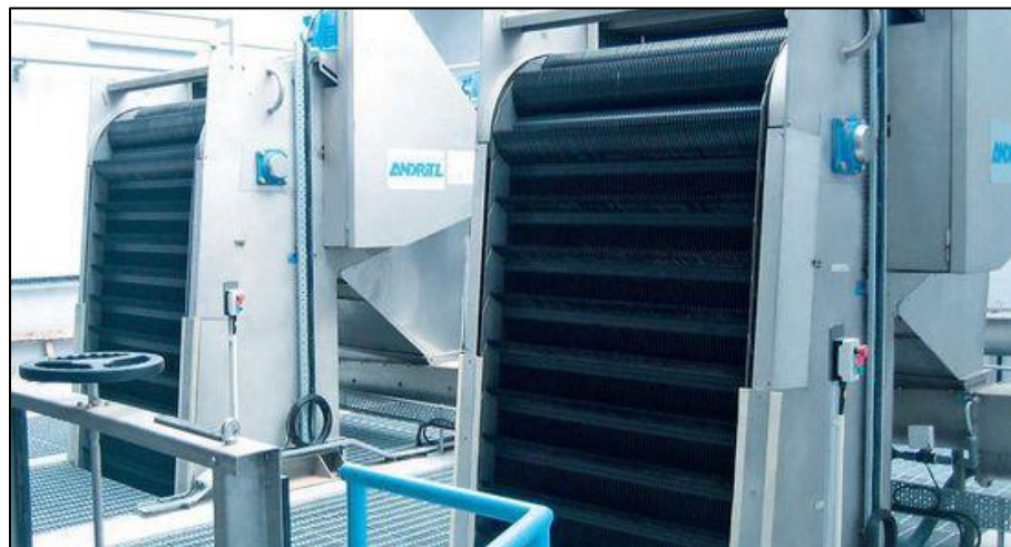
Figure 5. 3 Continuous Belt Bar Screen [24]
