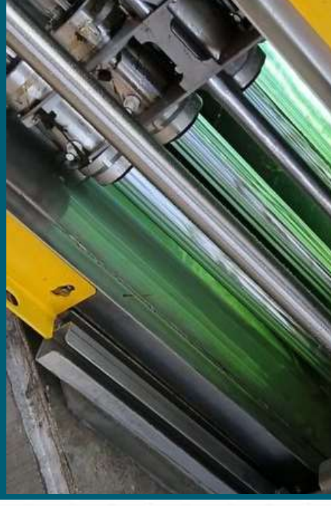
Figure 8: Trojan UV Signa Lamp Cleaning [8]
