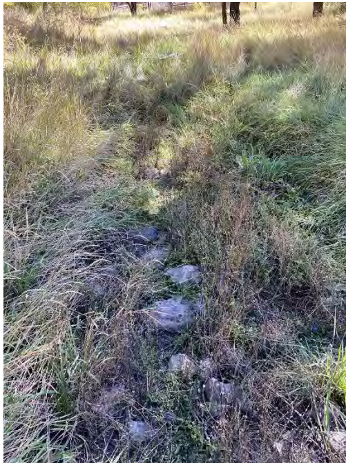
Figure 17: Station 2+80 Channel Debris
