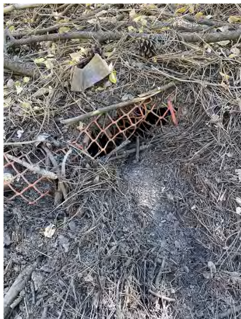
Figure 25: Culvert Inlet Obstruction
