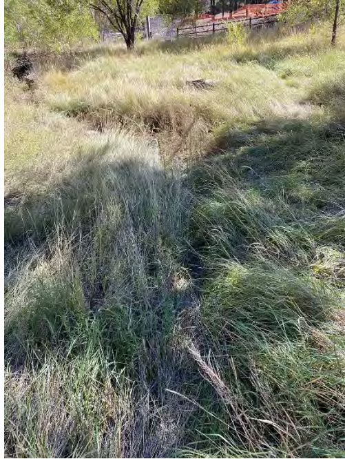
Figure 16: Station 2+80 Channel Overgrowth
