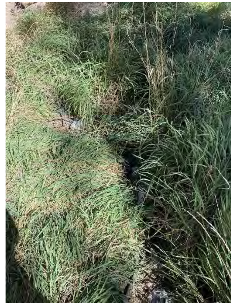
Figure 12: Station 2+10 Channel Overgrowth
