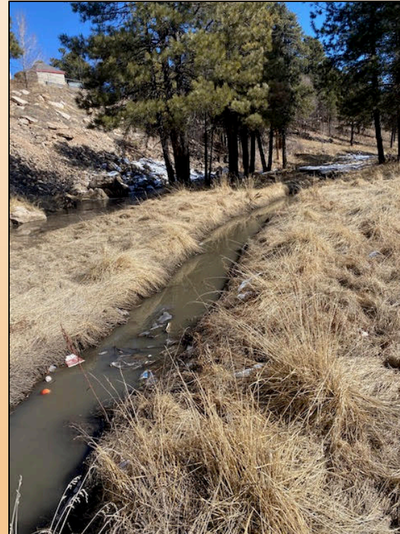
Figure 4: Ponding in Thalweg Upstream of Culvert
