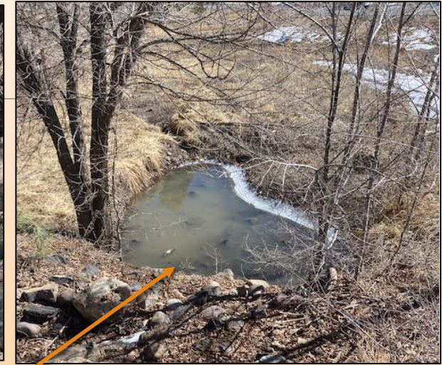
Figure 15: Scour Pool Ponding Culvert Outlet
