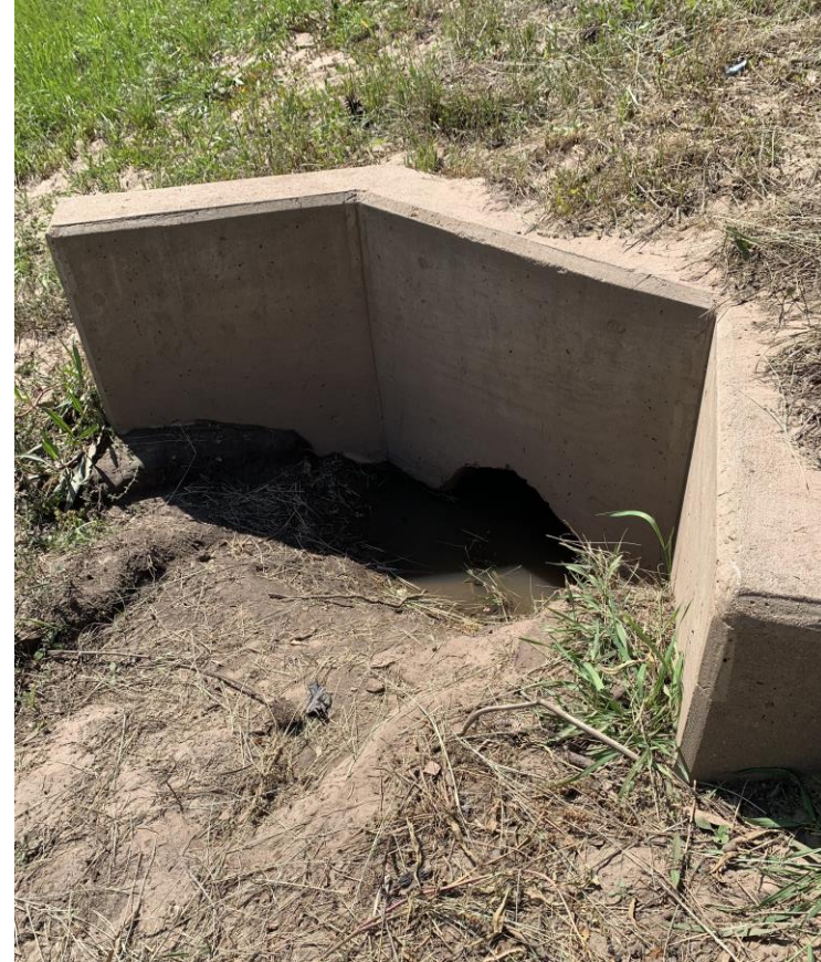
Figure 33: Detention & Silting at Culvert. Photo taken by Destiny Gourley.
