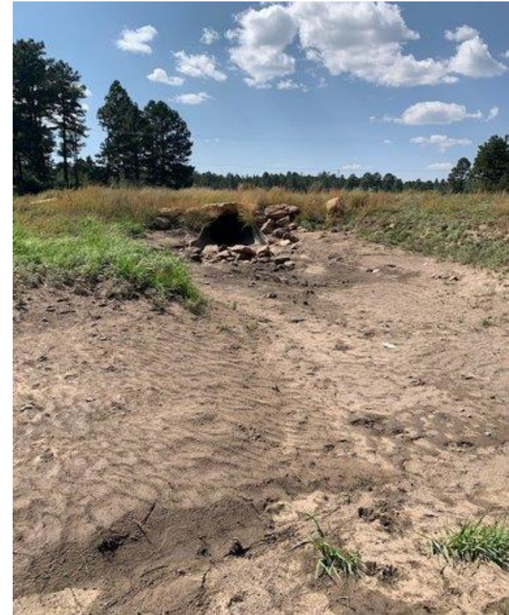
Figure 28: Rio de Flag channel station 44+06. This section of the channel shows detention and silting. Photo taken by Destiny Gourley.
