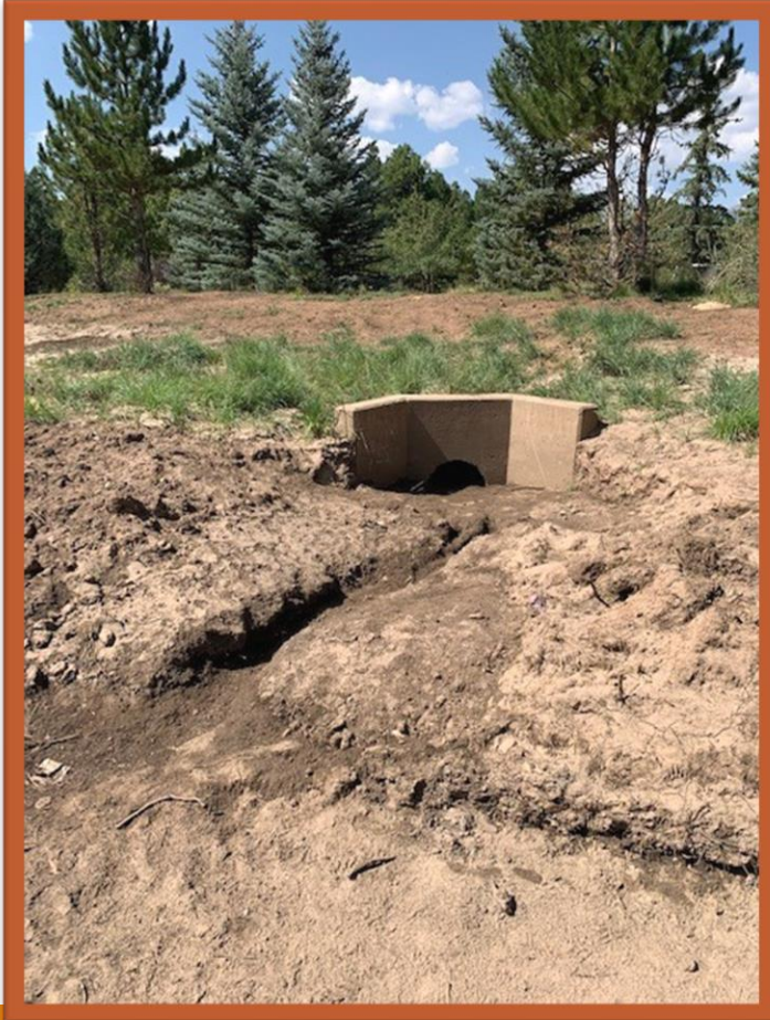
Figure 4: Rio de Flag channel station 71+84, looking west. Silting is present. Photo taken by Emily Frazer.
