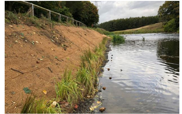
Figure 31: Erosion Control Blanket
