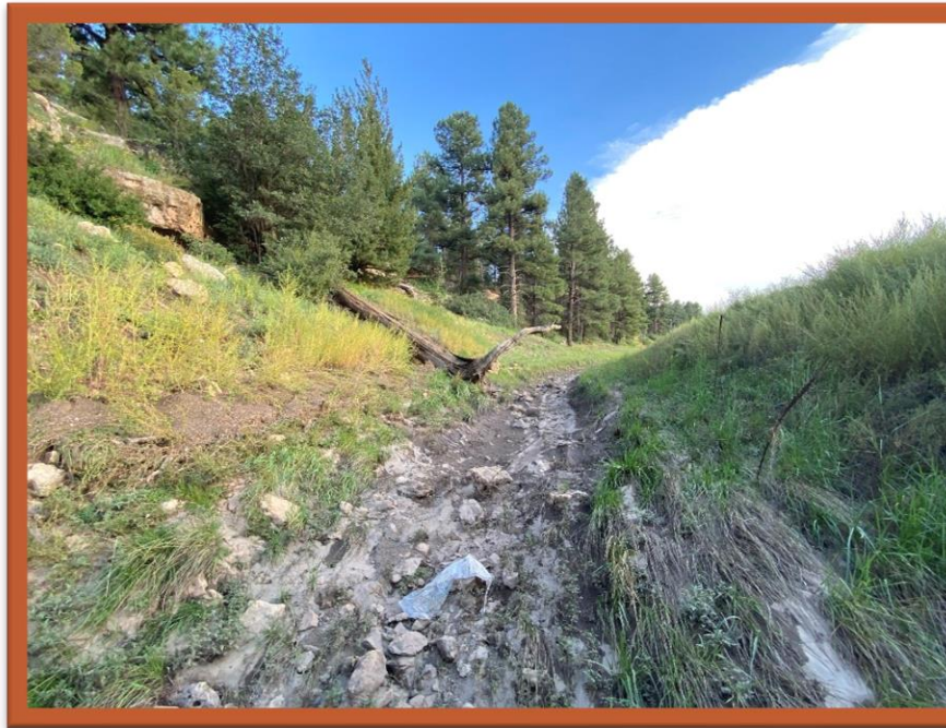
Figure 5: Rio de Flag channel station 60+13, upstream (south). This section shows garbage pollution within the reach. Photo taken by Jenna McCaffrey.
