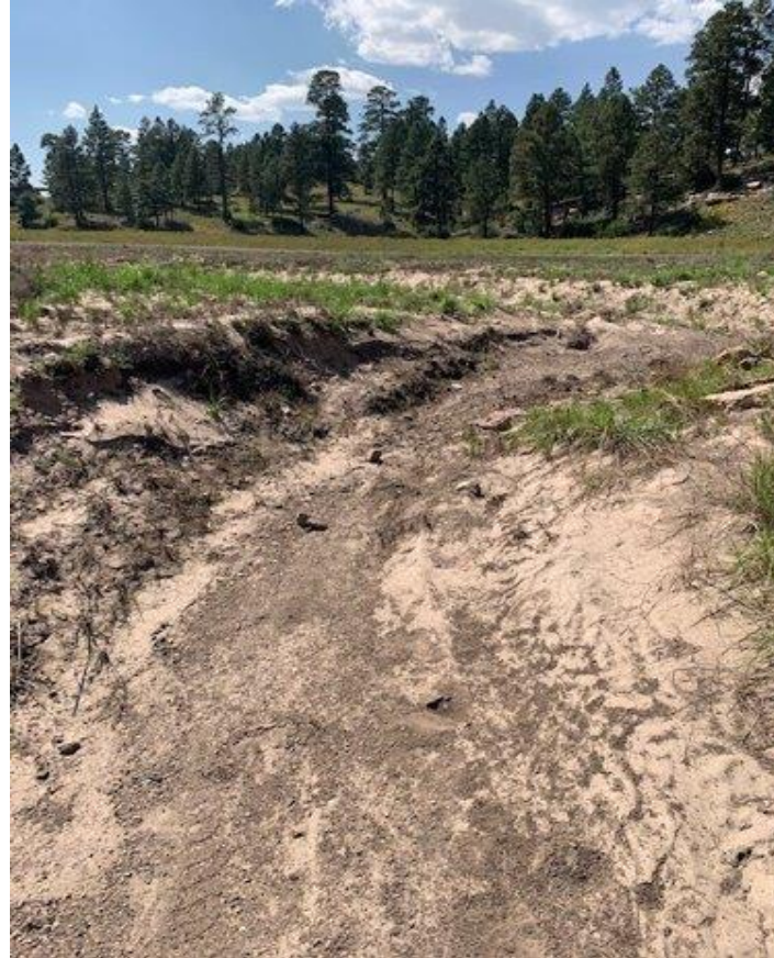
Figure 27: Rio de Flag channel station 54+77. This section of the channel shows erosion. Photo taken by Emily Frazer.
