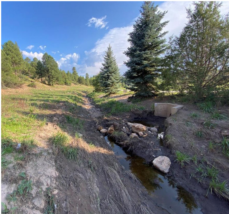
Photo Log 10: Rio de Flag channel station 78+87, looking upstream (south). Detention, erosion, and silting is shown.
