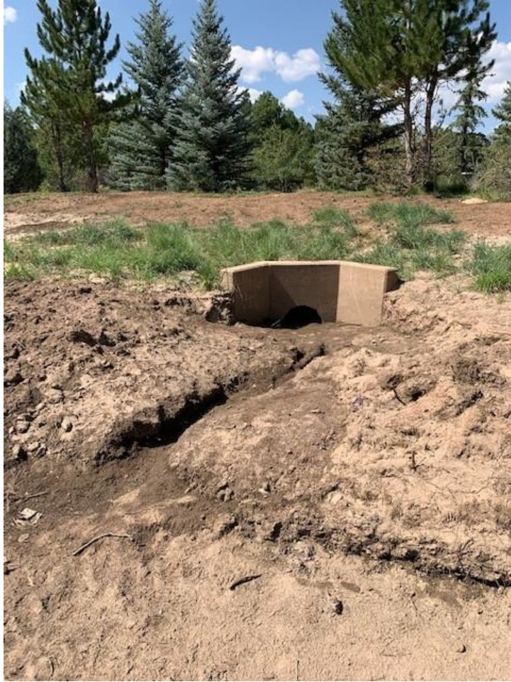
Photo Log 7: Rio de Flag channel station 71+84, looking downstream (north). Silting and erosion are present.
