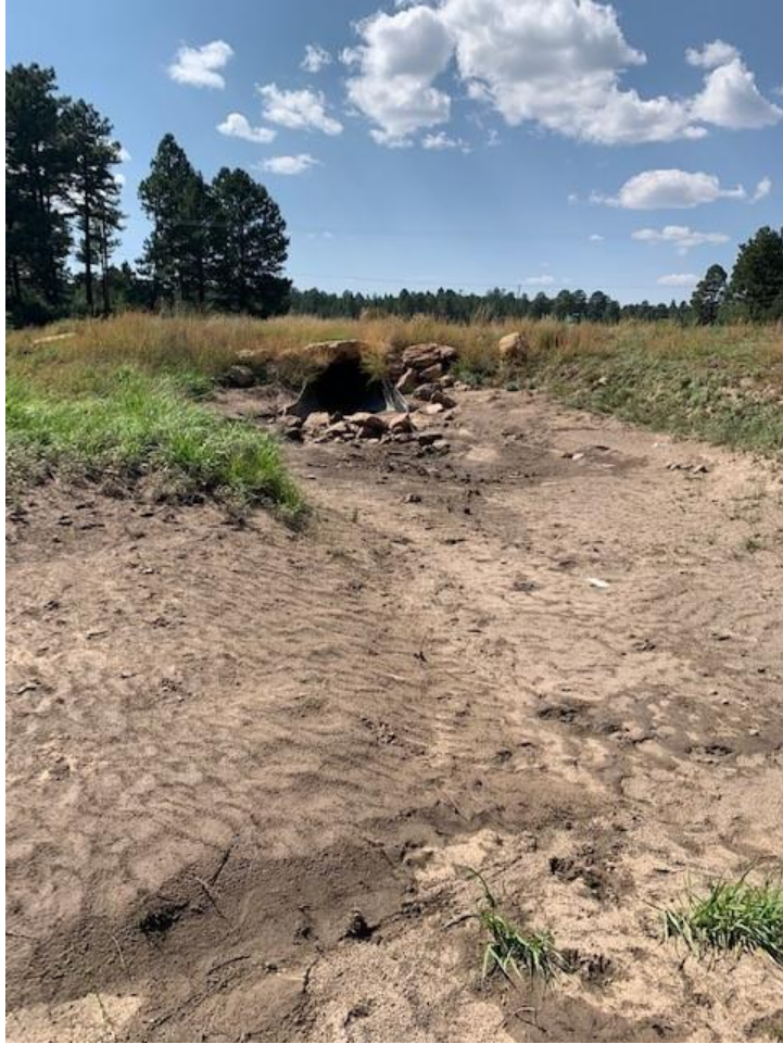
Photo Log 3: Rio de Flag channel station 44+06, looking downstream (north). This section of the channel shows silting and erosion.
