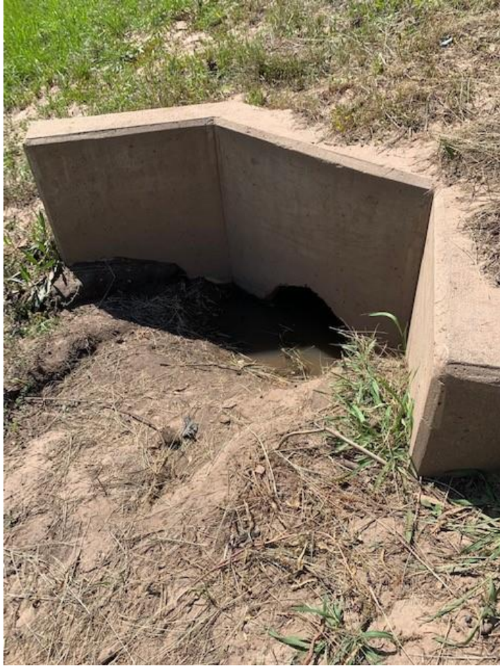
Photo Log 8: Rio de Flag channel station 76+97, looking downstream (north). This image shows silting and erosion.
