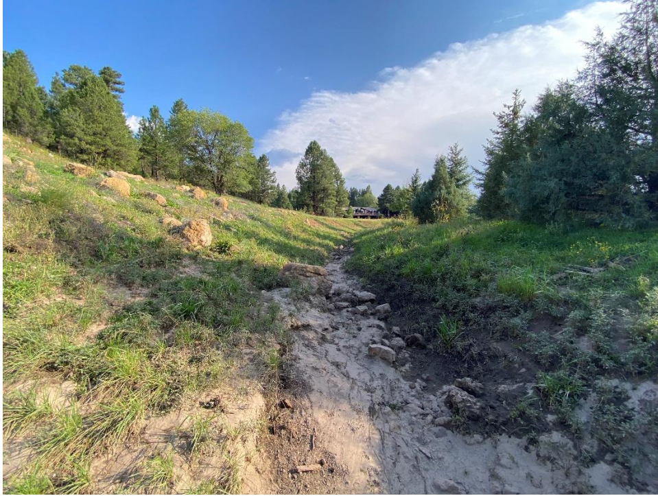
Photo Log 13: Rio de Flag channel station 82+60, looking upstream (south). This section shows silting and erosion.
