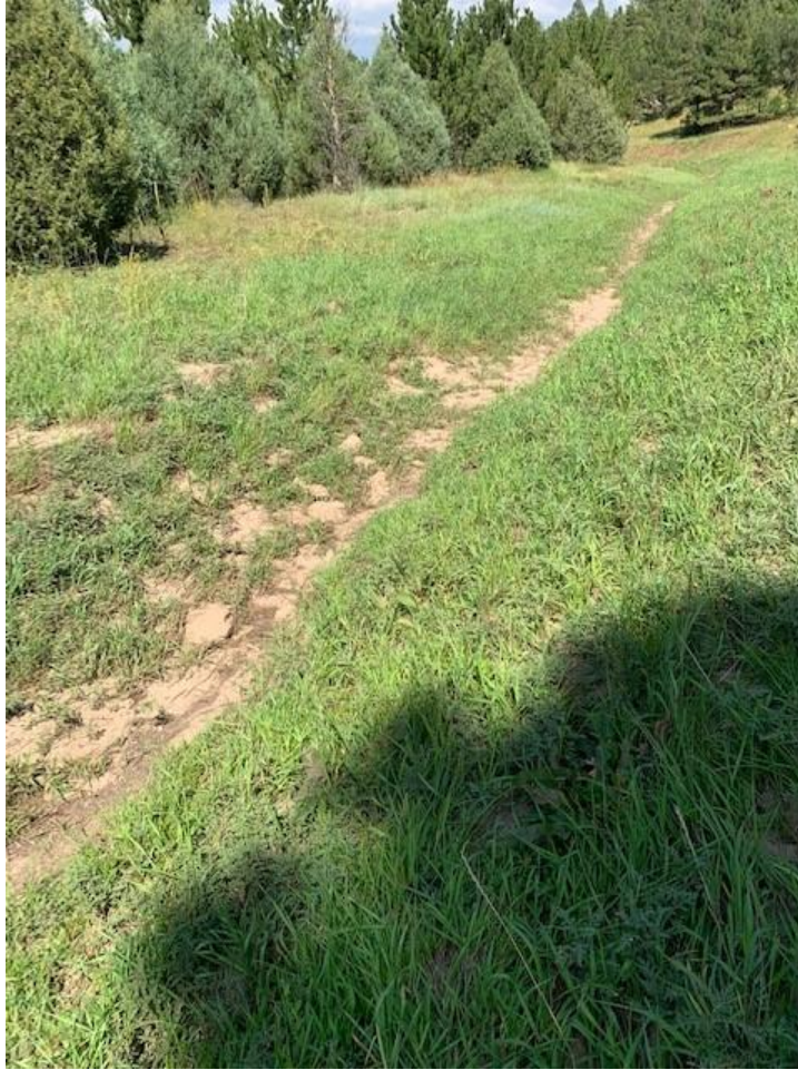
Photo Log 6: Rio de Flag channel station 70+09, looking downstream (north). This section of the channel shows silting, it is apparent that detention or retention would occur in this area had a flow been present.
