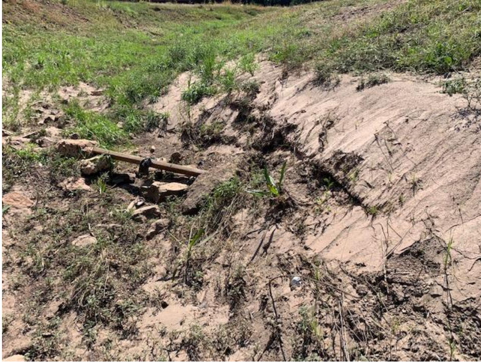
Photo Log 9: Rio de Flag channel station 78+15, looking upstream (south). This image shows silting and erosion.
