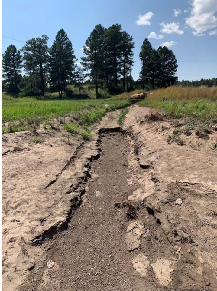
Photo Log 2: Rio de Flag channel station 37+10, looking upstream (south). This shows silting and erosion
