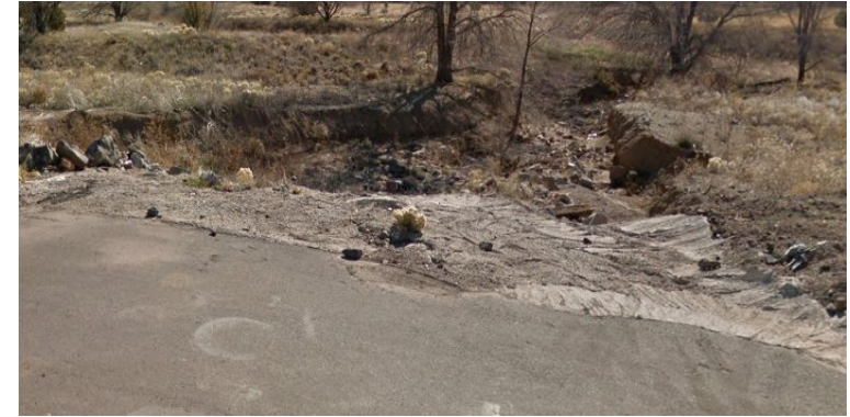
Figure 3: Erosion at Low-water crossing [1]
