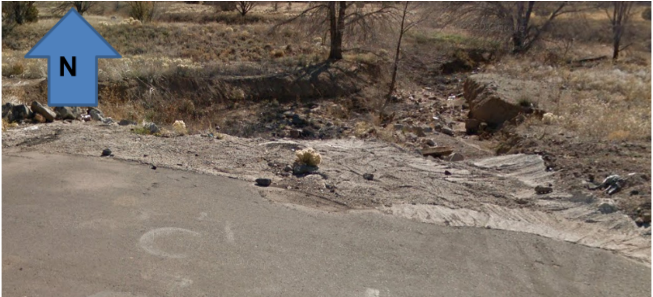
Figure 1.6: Erosion at Low-Water Crossing
