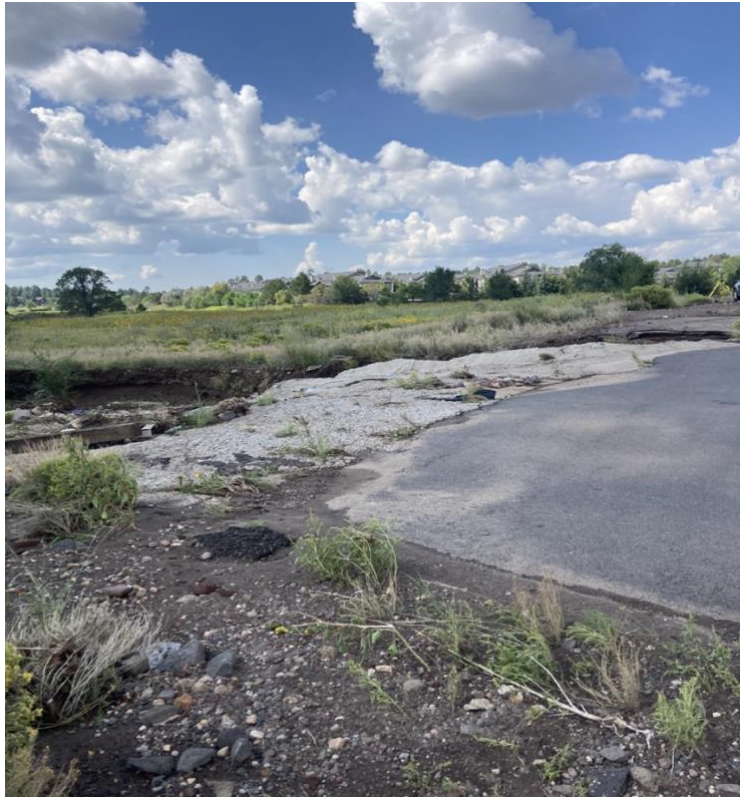
Figure 1.5: Erosion of Concrete above Rio de Flag
