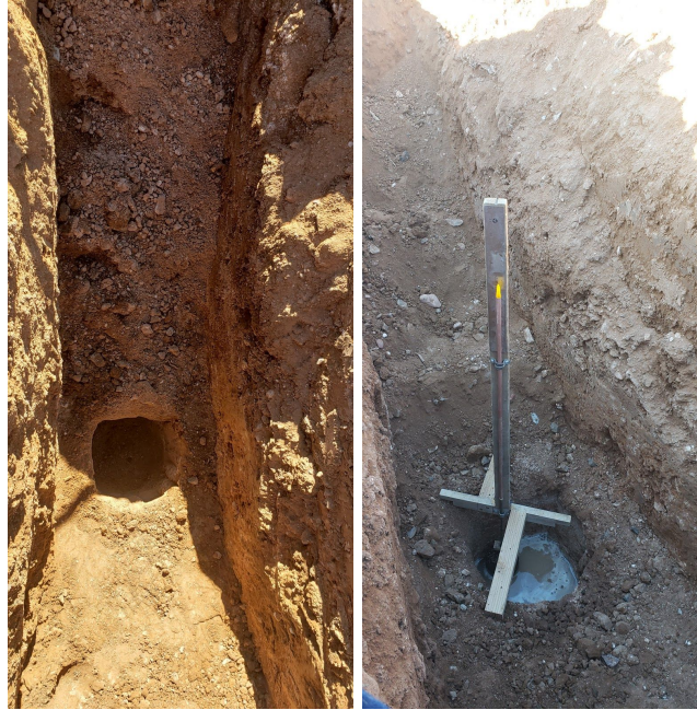
Figure 2: Typical test pit after excavation (right) and a test pit with ongoing infiltration test (left).
