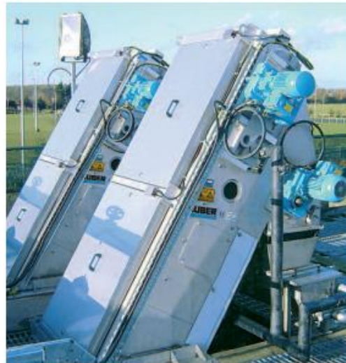
Fully enclosed for odor control
