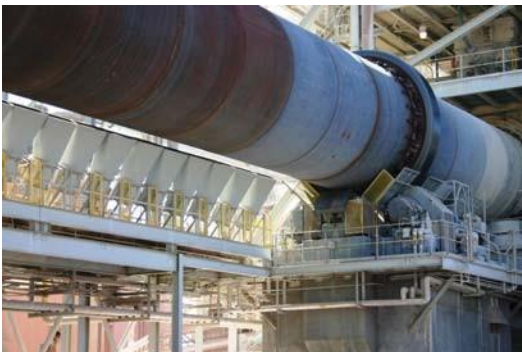
Cement Rotary Kiln, Clarkdale AZ
