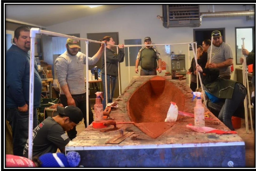
Figure 23: Once the final layer was placed on the canoe, PVC pipe was used to create a curing chamber around the canoe.
