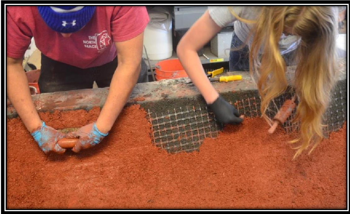
Figure 19: The finishing red layer is being carefully placed with the trowels and rollers onto the layer of reinforcement.
