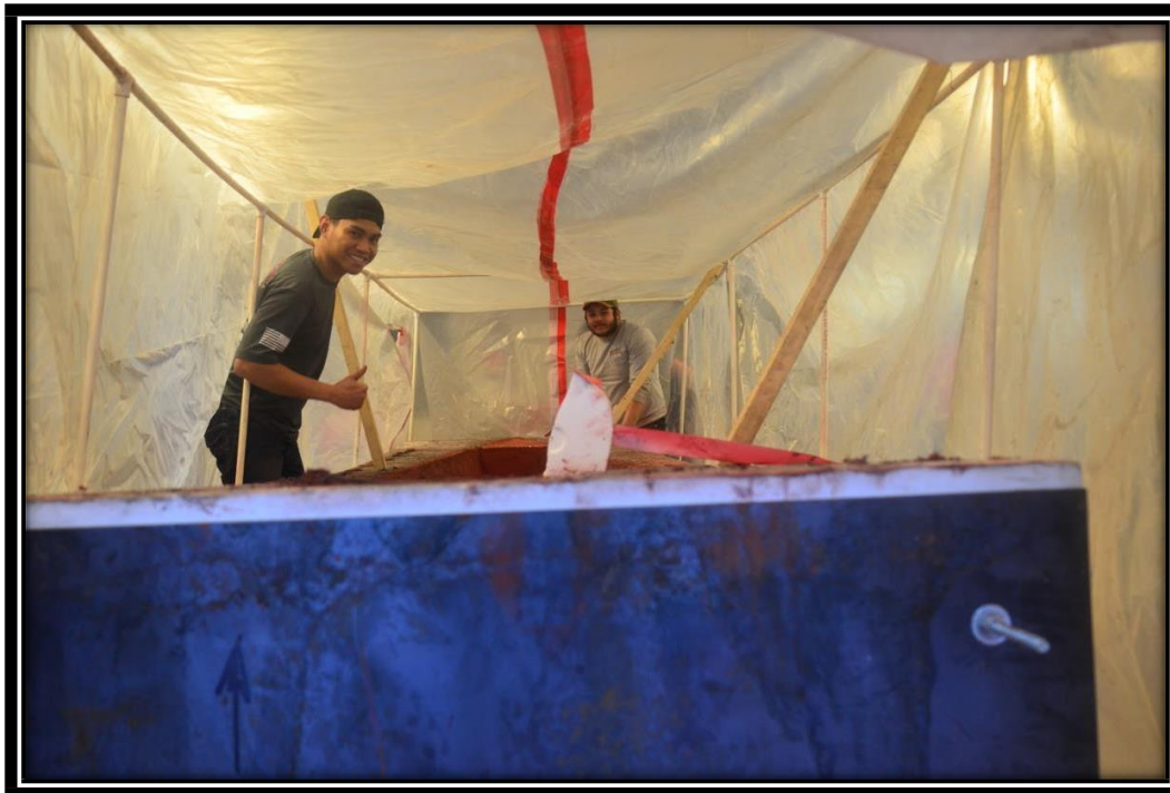
Figure 24: A plastic 6mm tarp was placed over the PVC pipe to avoid the escape of moisture.
