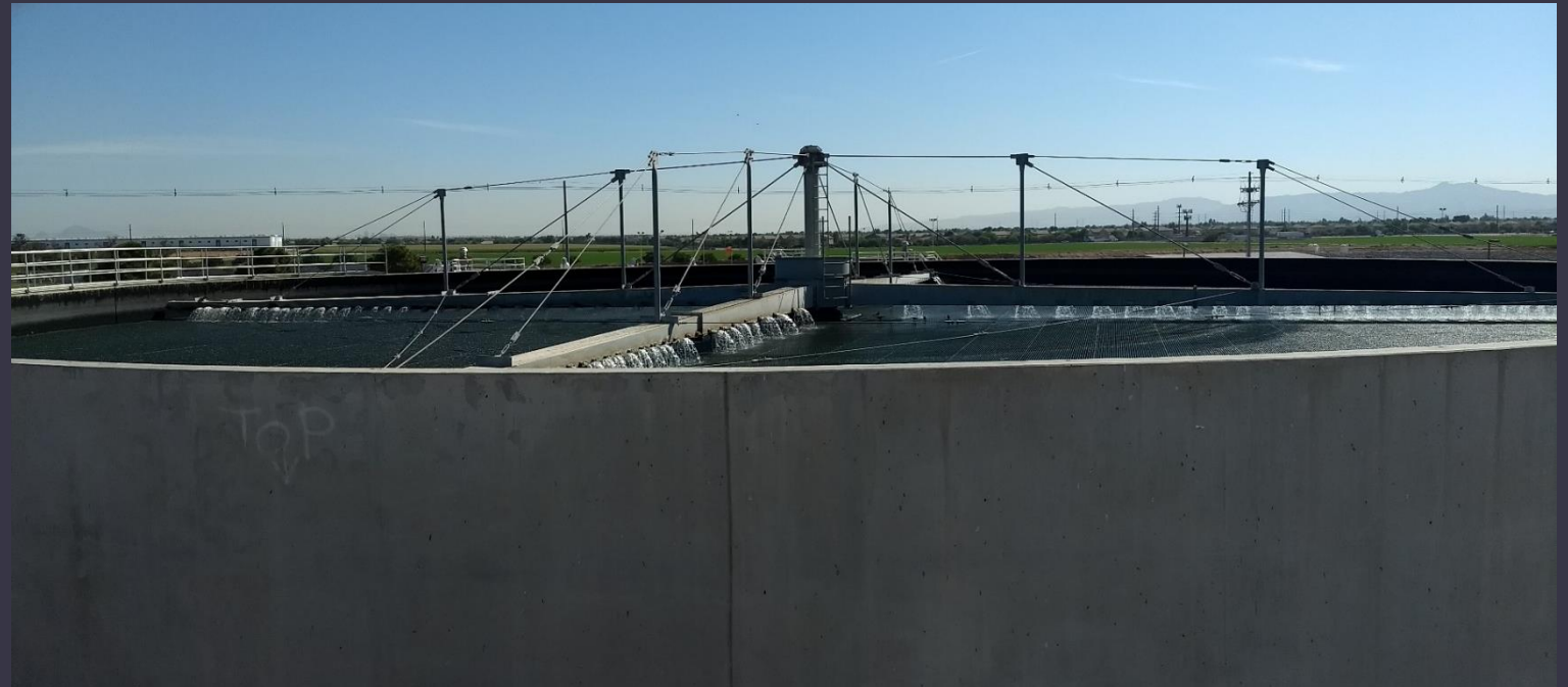
Figure 1: Tollesen WWTP Trickling Filter Photo by: Jed Ward
