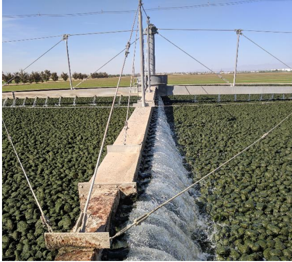
Figure 1: Tollesen WWTP Trickling Filter
