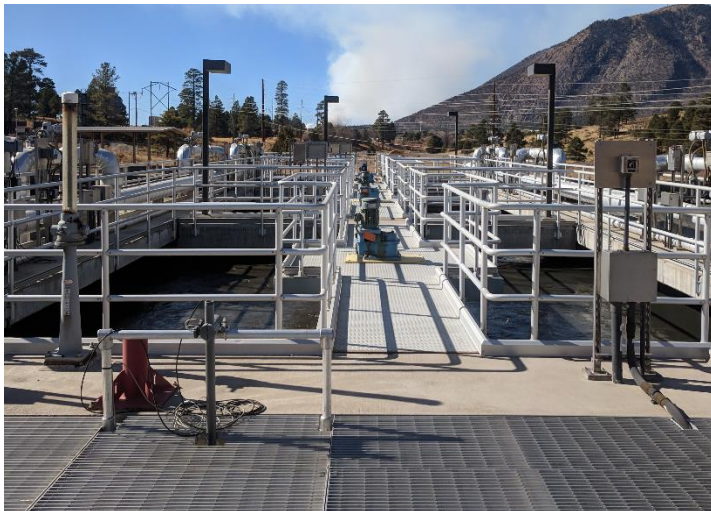
Figure 2: Wildcat WWTP Aeration Basin
