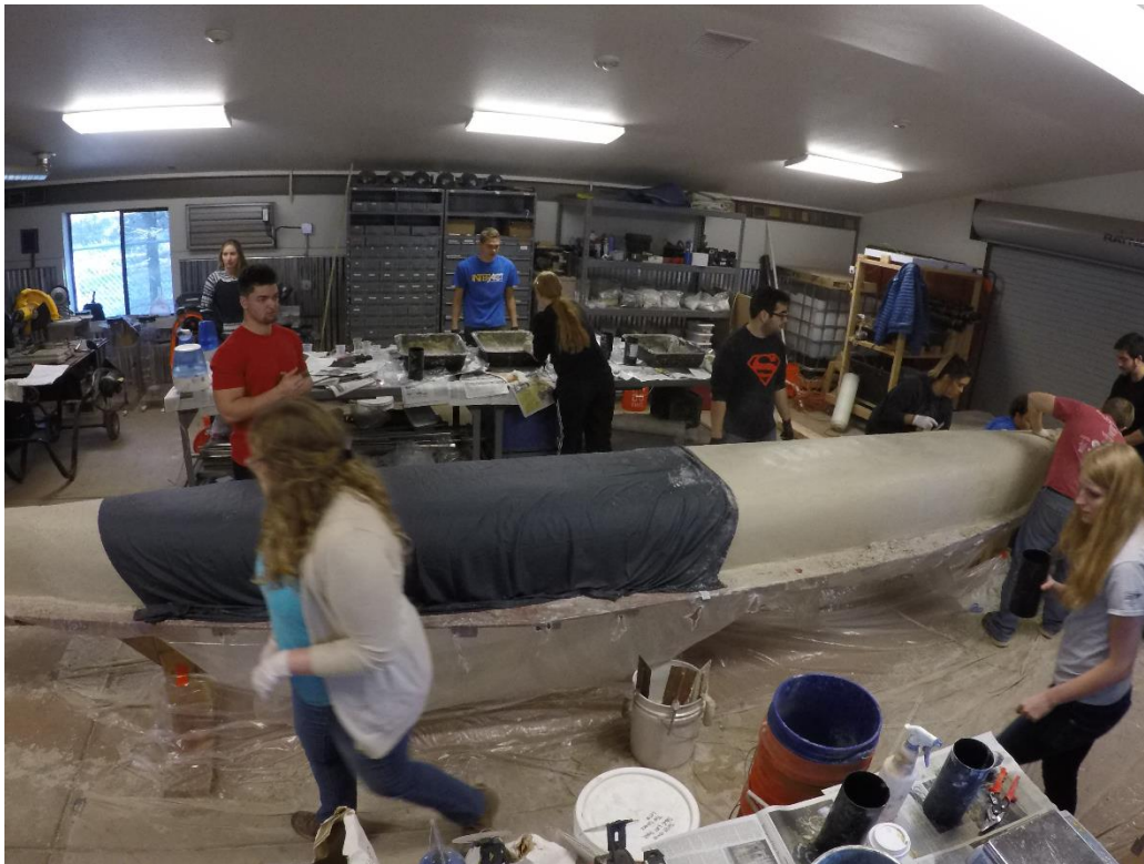
Photo 4. Preparing for First Primary Reinforcement: To keep the concrete moist, a damp cloth was placed over the area where reinforcement was not prepared to be placed.
