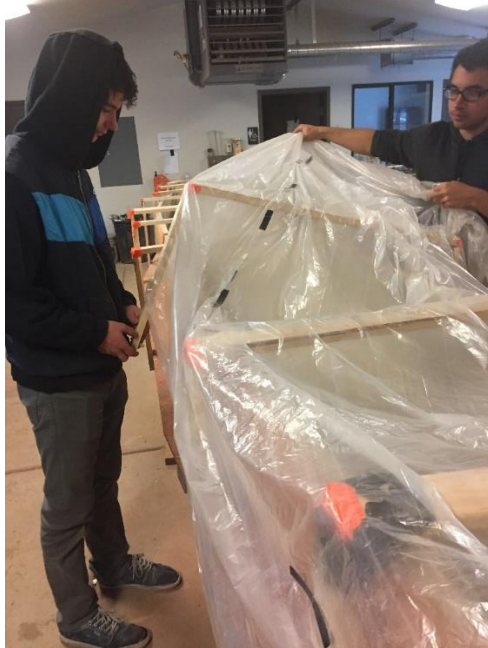
Photo 1. Curing Chamber Construction: Curing chamber was assembled with wood pieces that were inserted into holes on the sides of the construction table and a plastic tarp was used to encase the canoe. Allowing moisture to stay inside the chamber and properly cure.
