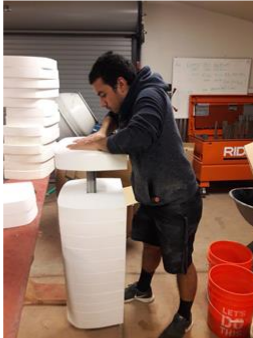
Photo 7. Preparing to Assemble Mold: Cross-Sections were put together with a 2 in. x 2 in. steel bar. This was done to keep the mold stable while applying concrete during casting.
