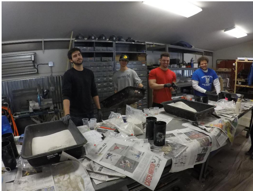
Photo 2. Mixing Station at Pour Day: Designated mixing stations were located next to the canoe. While casting was occurring, concrete was being prepared in four tubs with material that had been pre-batched.
