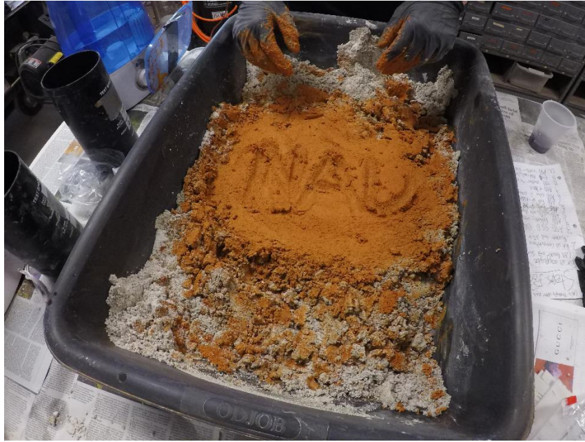
Photo 3. Mixing Concrete in Tubs: Finishing mix being prepared after the coloring admixtures had just been added.
