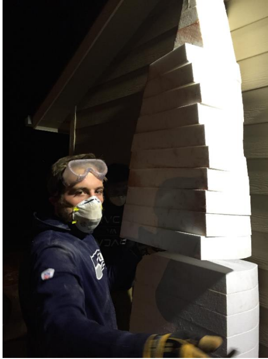
Photo 5. Organizing Cross-Section pieces to be cut: The foam cross-sections are arranged in the order and prepared to be cut with a hot knife foam cutter.
