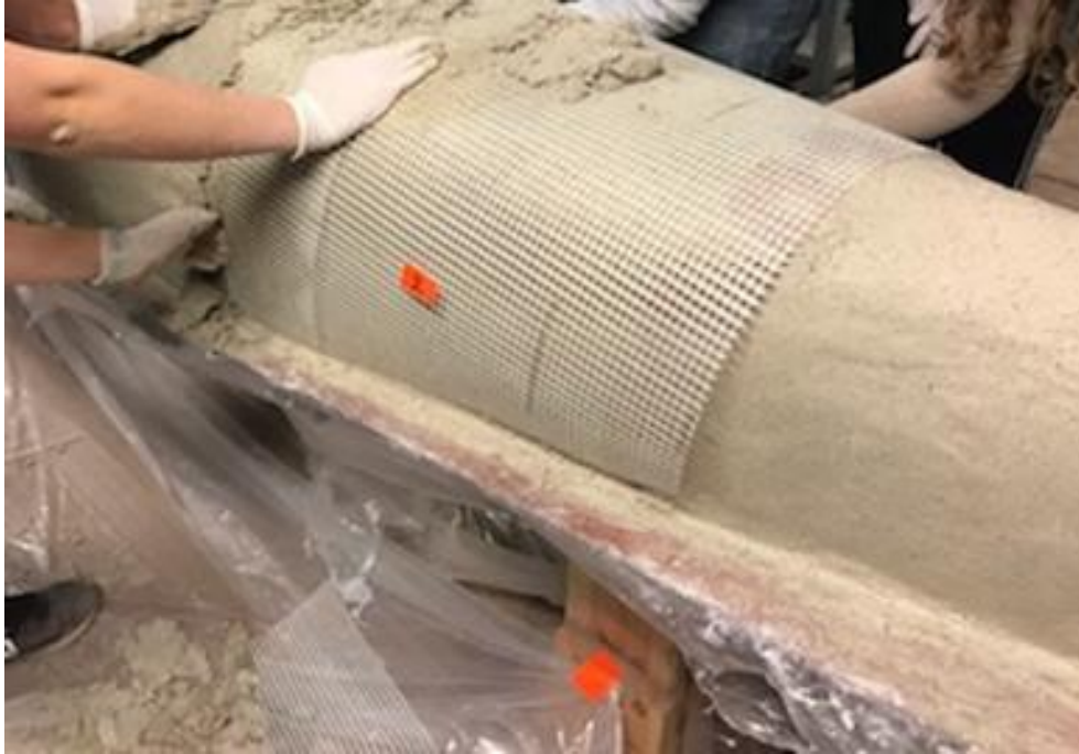
Photo 5. Placing Reinforcement Mesh: 11 sheets of mesh were used with 6 in. overlap to cover the full body of the canoe. Each layer reached from one side of the canoe to the other. Quality Assurance/Quality Control (QA/QC) was ensured by cutting the mesh to form to the canoe's shape.
