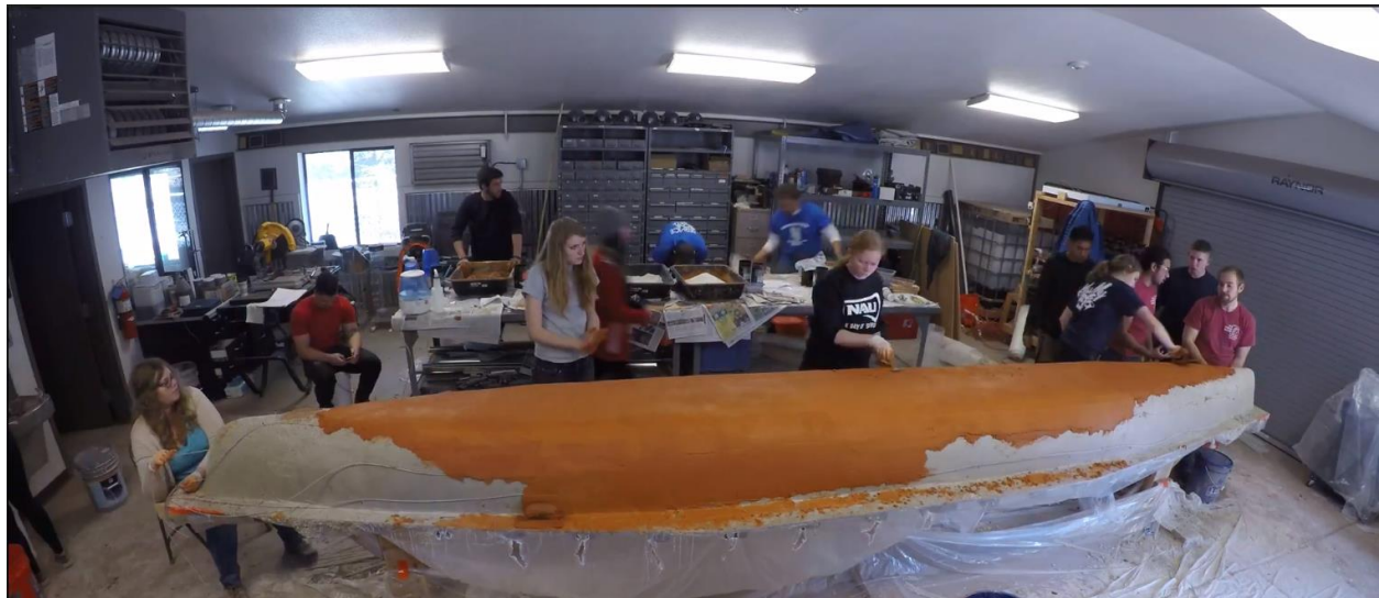
Photo 6. Applying Finishing Layer: The finishing layer was comprised of yellow and red admixture to create an orange color. The same application method of troweling was used. QA/QC was done using toothpicks that measured 1 ¼ in. deep.
