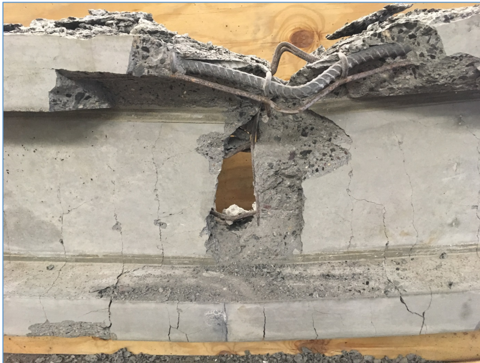
Figure 7.3.2 Condition of Beam After Failure
