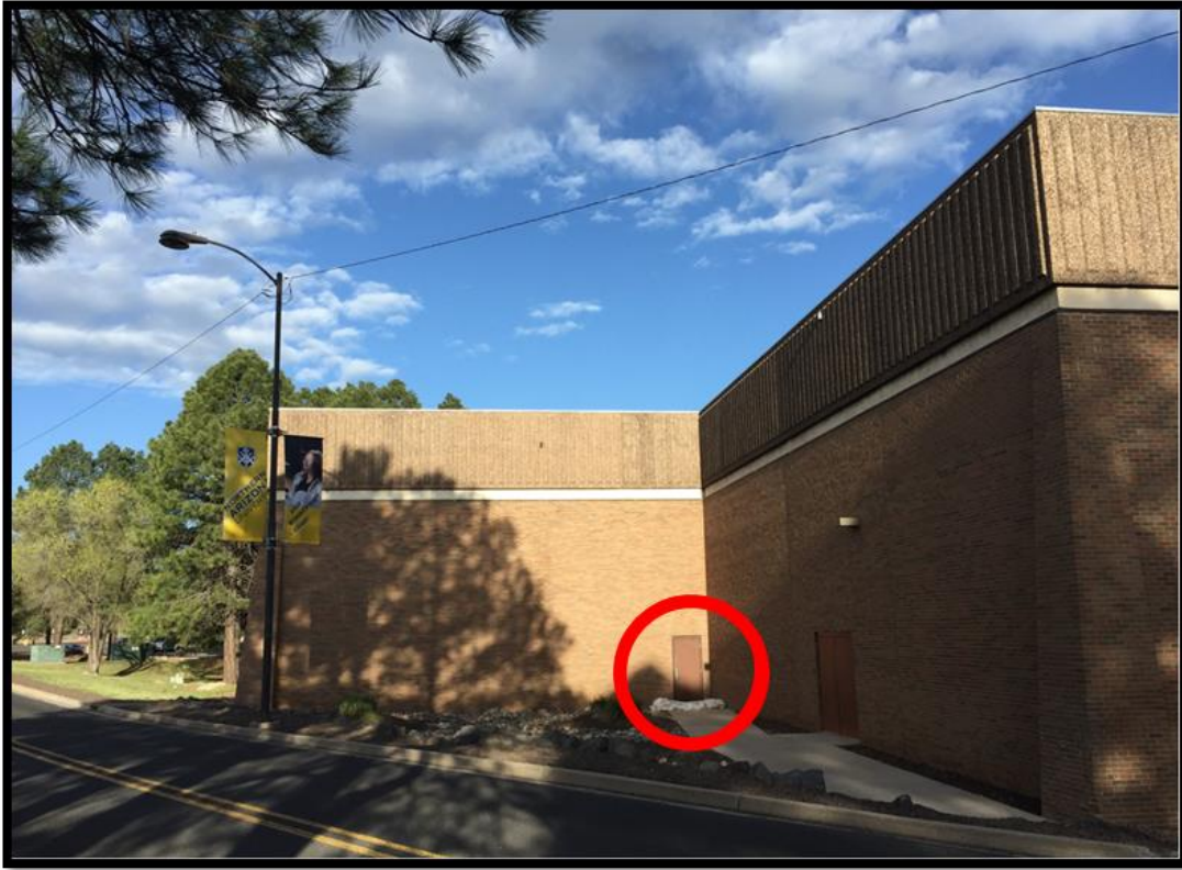
Figure 5. Flooding area behind Rolle Activity Center with sand bags on the Southeast door
