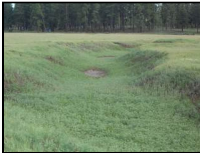
A ditch at Allan Lake 07/31/13
