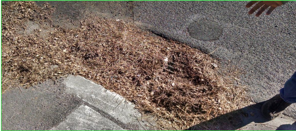
Figure 5-Clogged Storm Drains Surrounding Site
