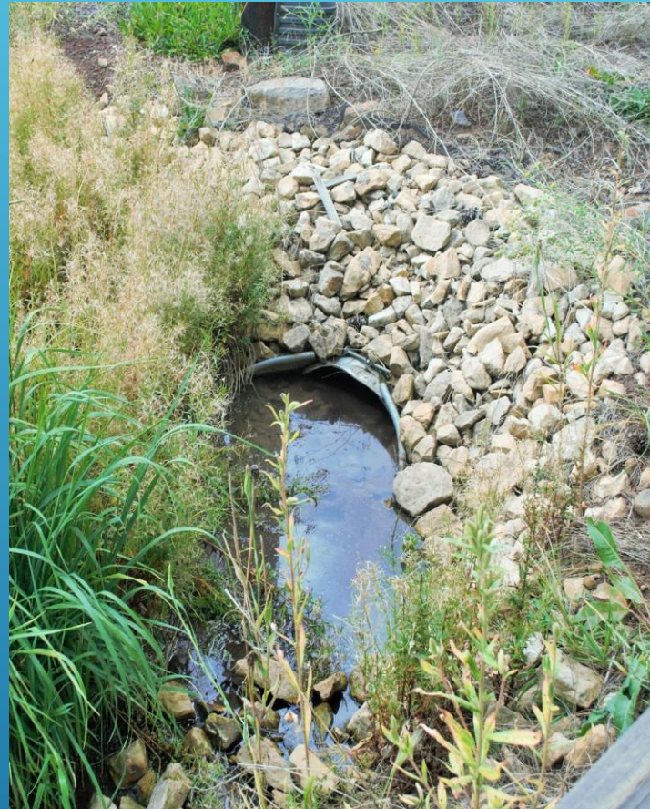
2ft Diameter Culvert Clogged By Sediment Due to Energy Fluctuations
