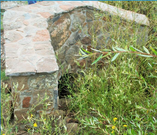
Left: Culvert Inlet Overgrown
