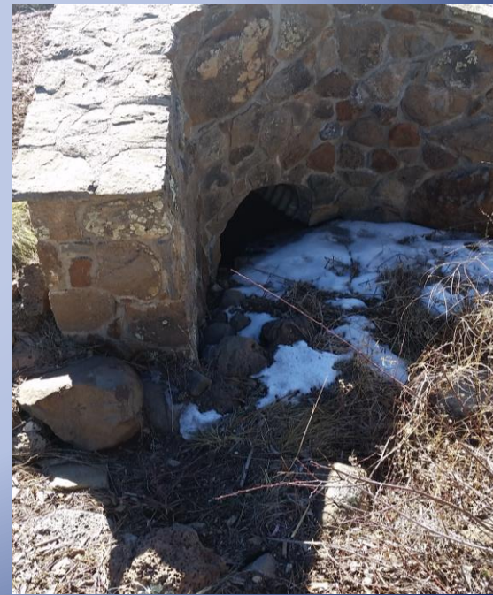
Culvert with Aggradation
