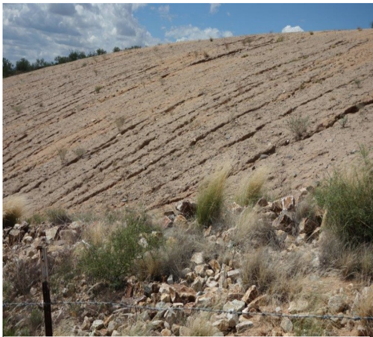
Figure 1.5: Vegetation is sparse and erosion is evident on the repository cap [5].
