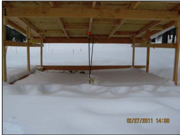
Figure 15: Possible contamination of the Roof 1 study plot
